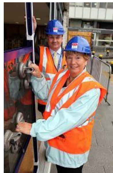
Mark Hopwood First Great Western's Managing Director and Plymouth City Council Leader Vivien Pengelly helping fit the new doors for the station
